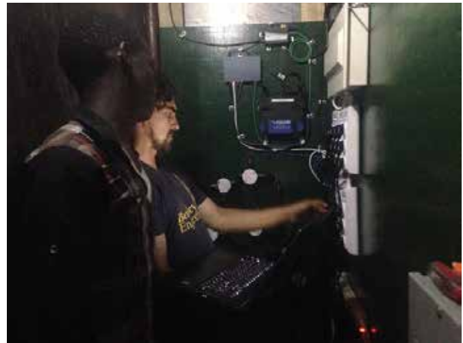
The Digi WR11 XT provides a reliable connection to the global 3G network while withstanding high operating temperatures of the network utility hub.
